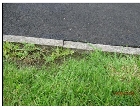
(Potential trip hazard at edgings)
