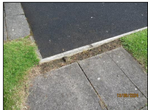
(Potential trip hazard at edgings)
