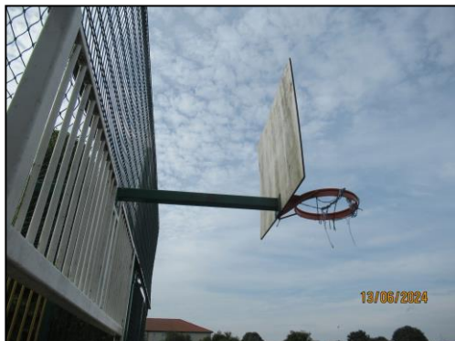
(Missing basketball back board frame)
