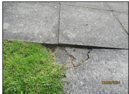
(Potential trip hazard at slabs adj to seat)
